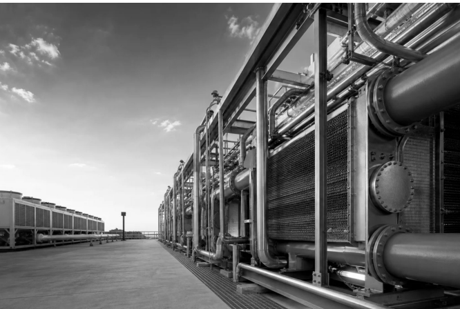
ENGINE & GENERATOR COOLING
