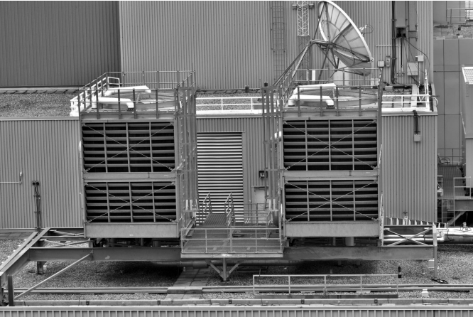
HEAT REJECTION & HEAT RECOVERY
