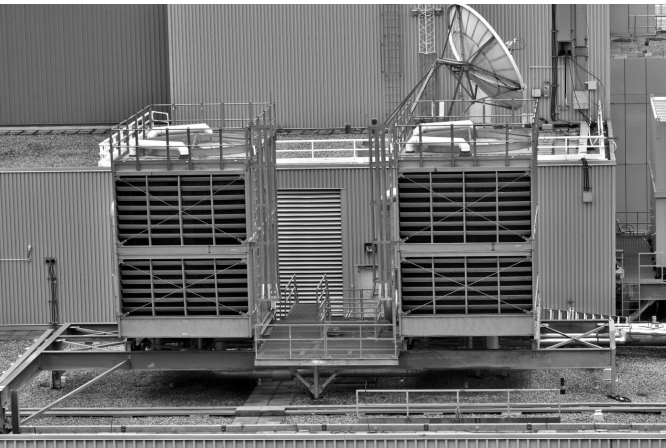
HEAT REJECTION & HEAT RECOVERY
