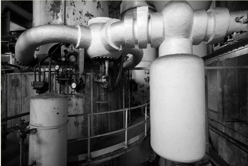
INDUSTRIAL BOILER AND PROCESS PIPEWORK
