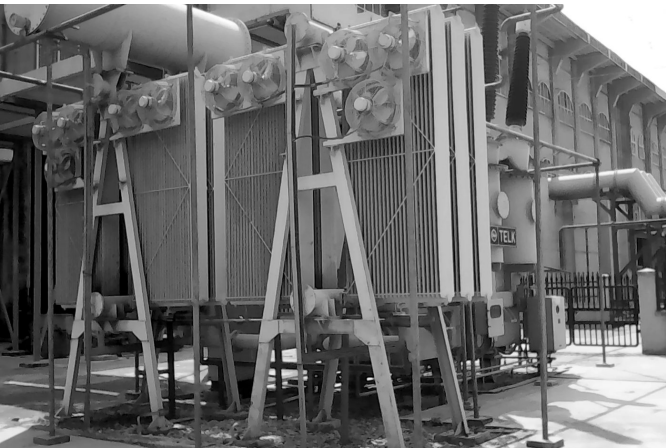
TRANSFORMER COOLING SYSTEMS
