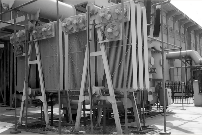
COOLING FANS ON A POWER TRANSFORMER
