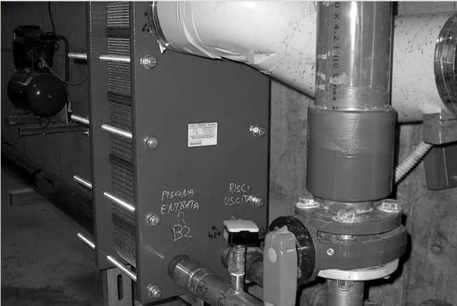
PLATE HEAT EXCHANGER INSTALLED IN A PLANT ROOM
