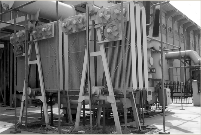
COOLING FANS ON A POWER TRANSFORMER
