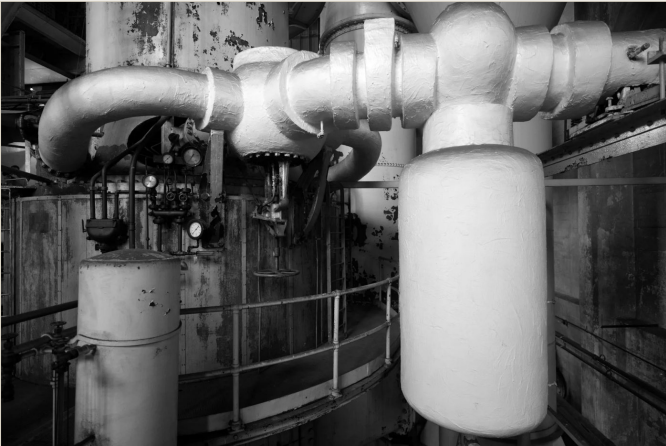
INDUSTRIAL BOILER AND PROCESS PIPEWORK
