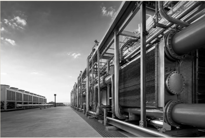
REPRESENTATIVE EQUIPMENT / OPERATING CONTEXT
